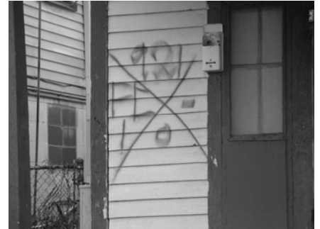
One of the many still uninhabitable homes in the 9 th Ward
